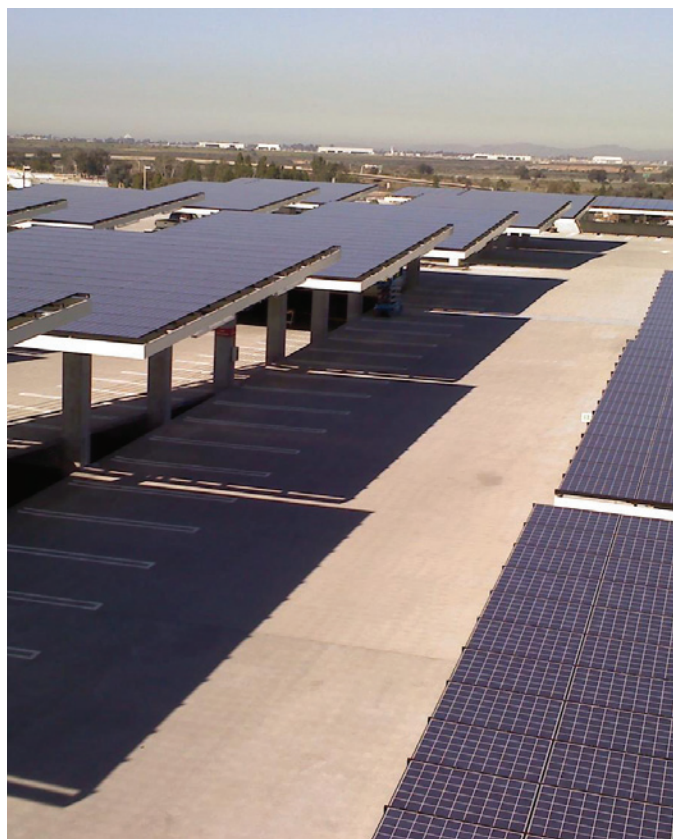
The SDG&E-owned 359 kW photovoltaic system on the roof of one of the parking structures provides enough clean, renewable energy to power over 200 homes in San Diego. Photo by Independent Energy Solutions.
